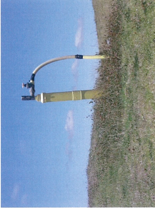
Gas extraction wells
