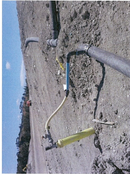
Gas Collection Pipework
