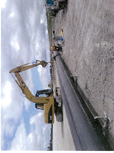
Main Gas Header
