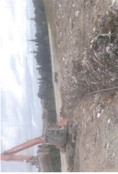
Gas Well Laterals
